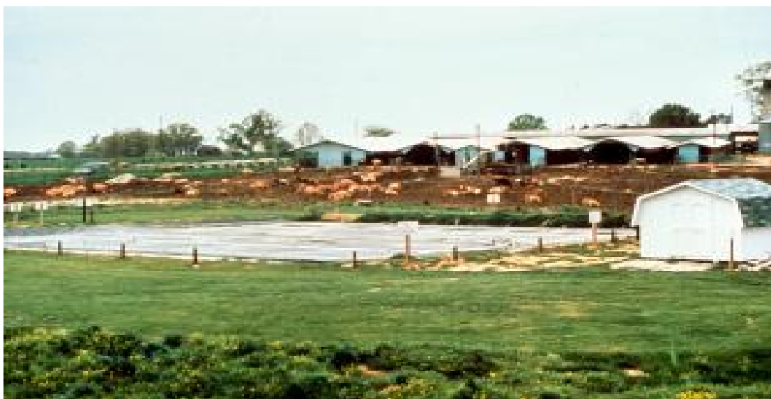
Figure 8. Covered lagoon system at Randleigh Dairy (photo credit: RCM Digesters)
